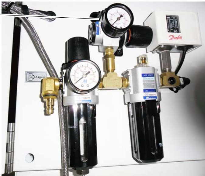
Img.10-5: Compressed air service unit
