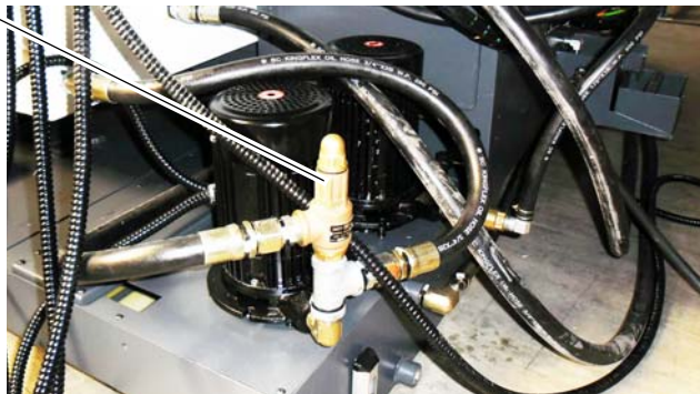
Img.3-10: Coolant / lubricant pumps
