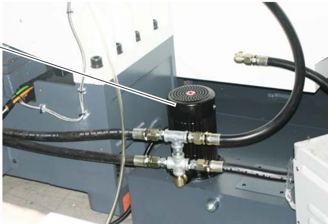
Img.3-11: Coolant / lubricant pumps
